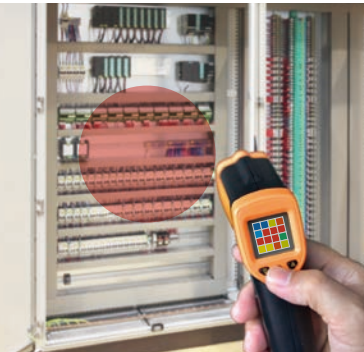
Transformers & distribution boards
